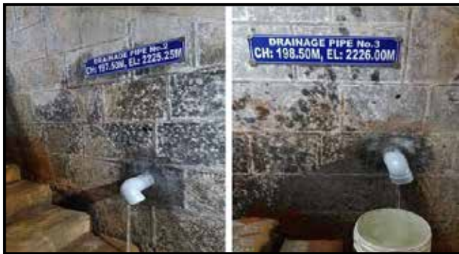
Fig. 9 : Drainage Pipe from behind the geomembrane exiting into the gallery to collect any water that is accumulated behind the membrane
