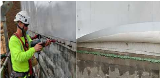
Fig. 10 : Installation of Perimeter seal. Resins and bedding mortar seen before placing the perimeter seal
